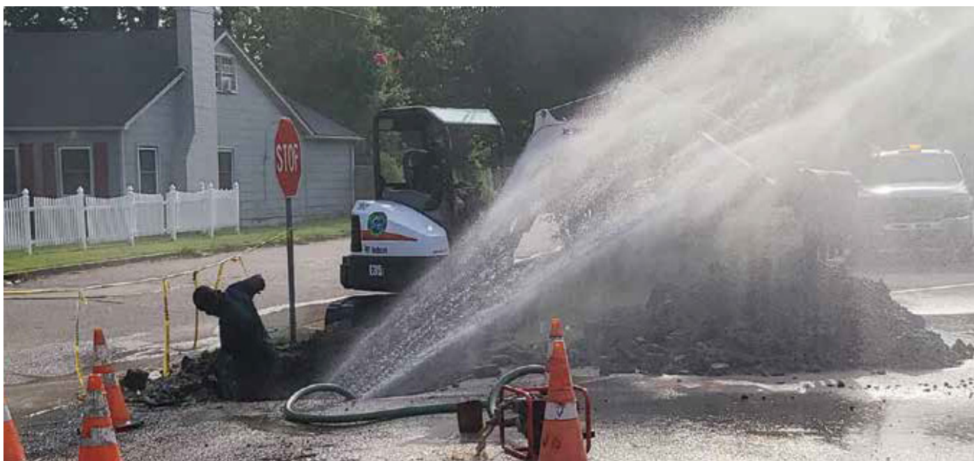
Greenville alerted to leak on 16-inch water main through ASTERRA Recover program. Photo courtesy of David Hangar, Water Maintenance Division, City of Greenville.
