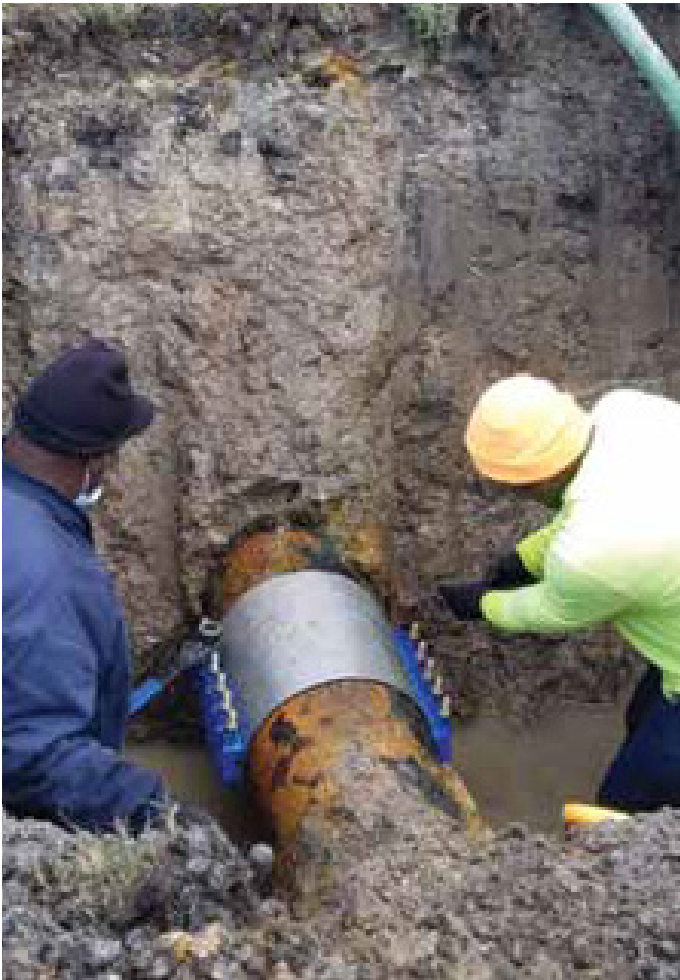
Greenville crew repairs leak that would likely have gone undetected. Photo courtesy of David Hangar, Water Maintenance Division, City of Greenville.
