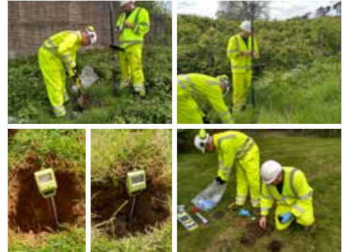
Figure 3. Crick: top left to right - excavating topsoil, taking coordinates with Trimble RTK. Bottom left to right – measuring water content with soil moisture probe, sampling soil.
